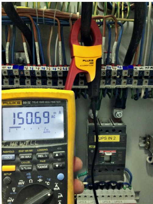
9. Testing system max current load on half of the audio system during commissioning. (150A)
