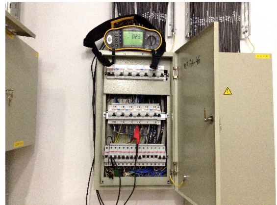
10. A common multi-function installation tester can be a useful diagnostic tool.
