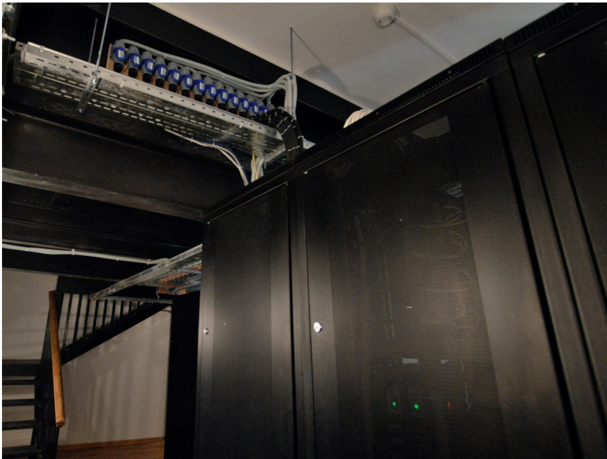
4 Equipment rack fed with 13 x 16A lines each on 6mm cable where high power equipment shares rack space with IT and sensitive audio systems. That's a lot of copper back to source.
