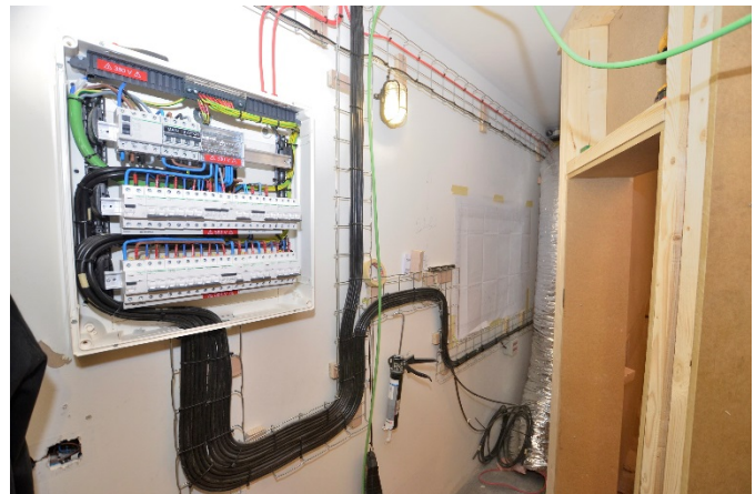
6. A local sub-distribution board in a recording studio service area under construction providing a local radial topography that will match the audio installation layout. (Barcelona)
