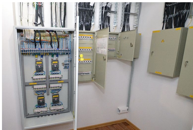
3. 500A (2 x 250A) Audio / Video systems only power room for a film post production studio (CP Productions / NTV Kino – Moscow)
