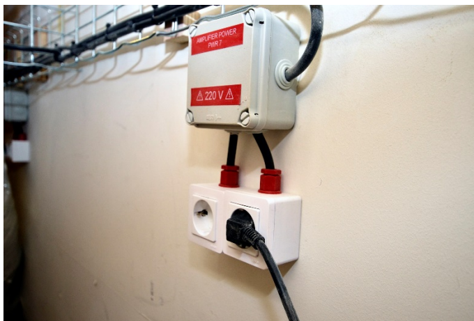
7. A 6mm cable fed from 16A breaker supplying two European 16A power outlets for the audio amplifiers in a recording studio. A terminal box is required to terminate the 6mm cable into the domestic sockets via 2.5mm short links.
