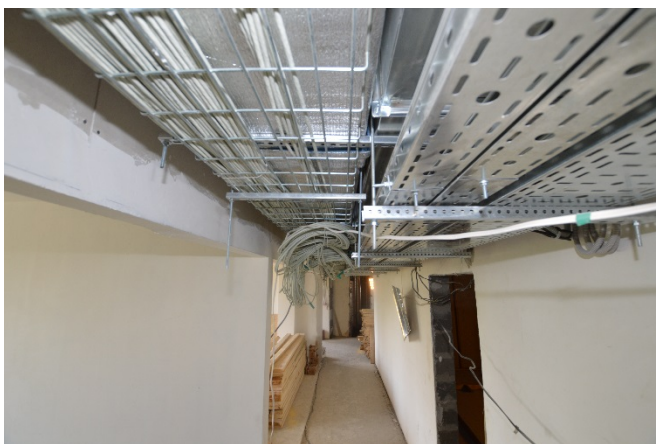
5 All technical service cables in a film post production complex following a common route with minor segregation distances to avoid creating a loop in the ground conductors.
